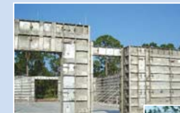
Aluminum forms are part of the solid poured concrete homes construction process.
